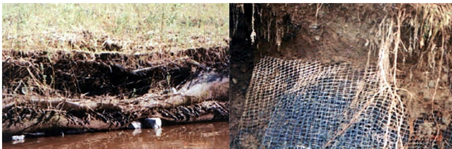
Failed vegetated soil-lifts (Alaska DOT FHWA-AK-RD-03-03 report)
